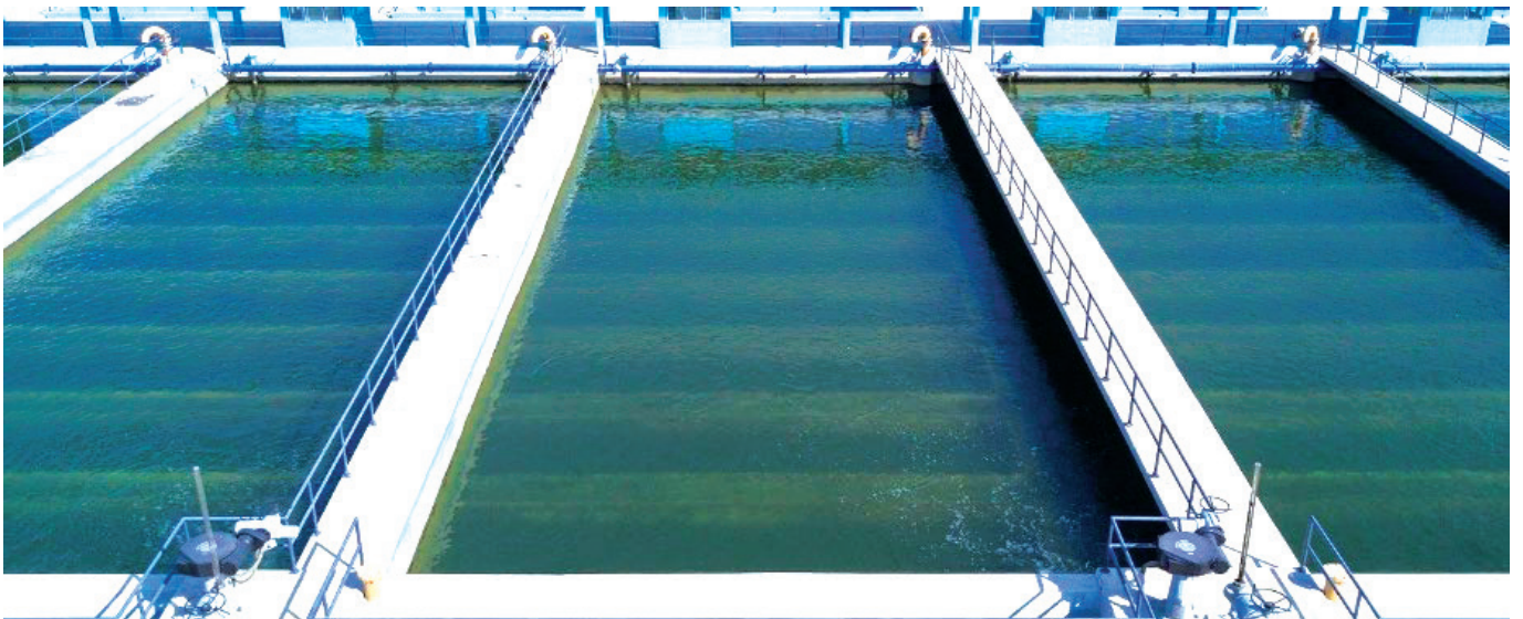
Rapid Sand Filter
