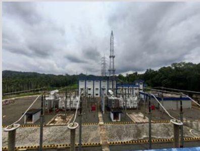
State's first 400kV Gas Insulated Substation (GIS) at Kuravilangadu, Kottayam
